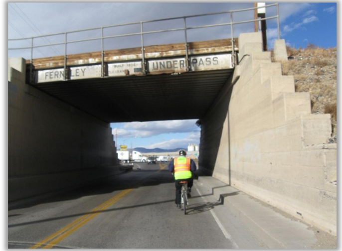
Fernley: Narrow underpasses can become pinch points for bicyclist, providing little room for shared use of a roadway segment.
