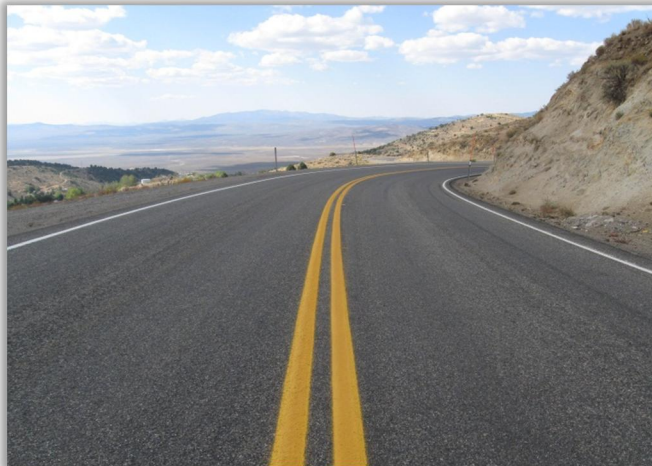
US 50, East of Austin: Narrow shoulders and blind curves
