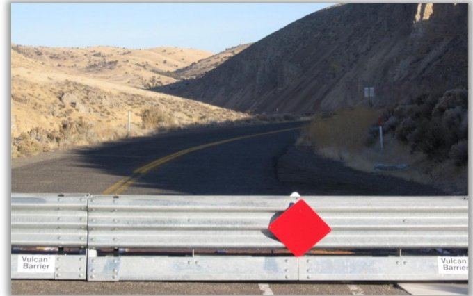
I-80, East of Carlin Tunnel: Old Highway available as alternate route
